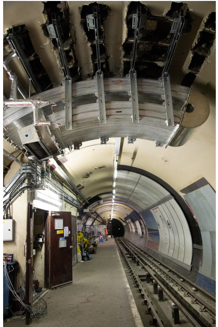
Trialling the system at a disused platform within the deep Tube environment
